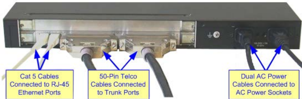
Figure 5-3: Cabling for 16-Span Device using Telco Connectors
